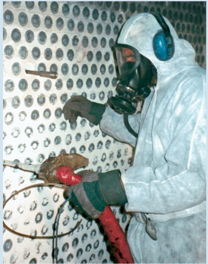
In some cases, gas masks are highly recommended – e.g. when cleaning heat exchangers and wherever harmful materials are blasted loose.
